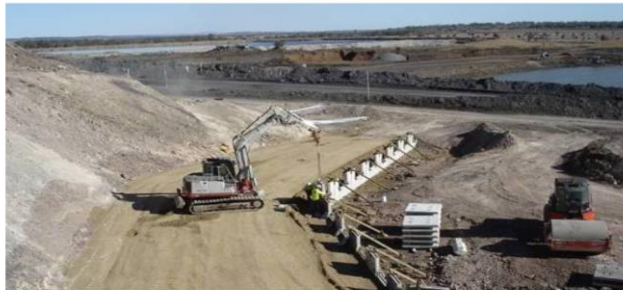
Work carried out at the New Acland mine site on Queensland's Darling Downs.
